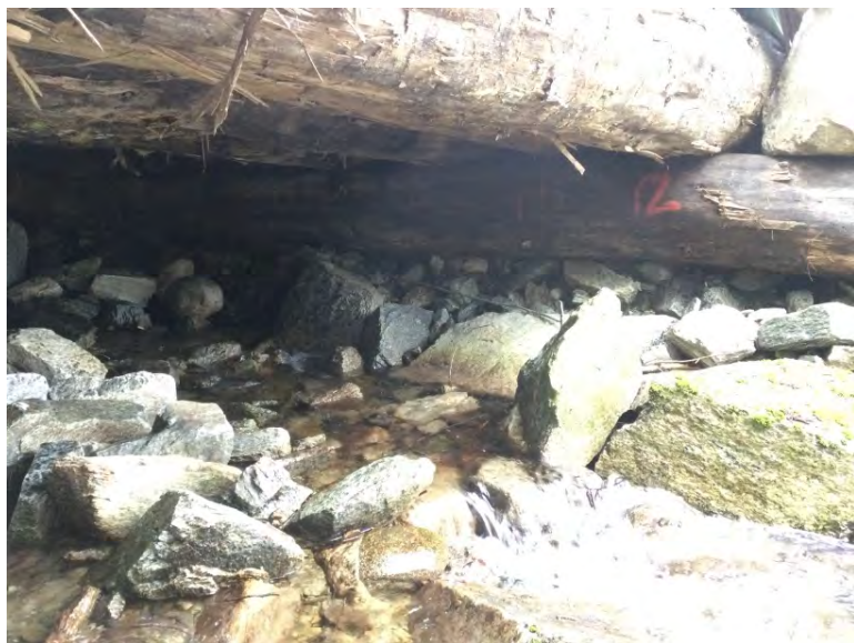
Erosion downstream left bank extends to stringer 7
