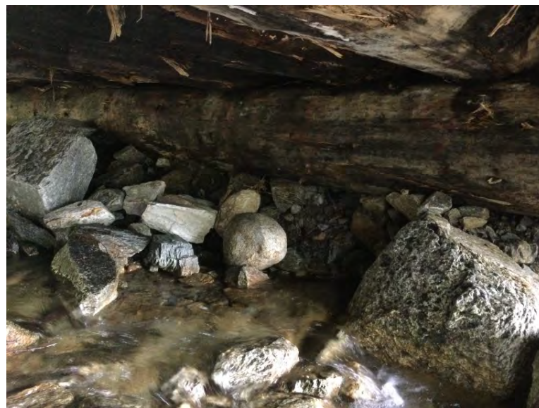
Erosion under stringers 7 and 8
